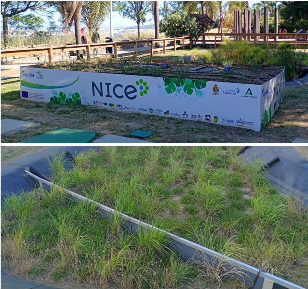
Figure 2.3.10 Installation photo of the storm water run off storage tank (top) and wetland basin for storm water treatment (bottom).
